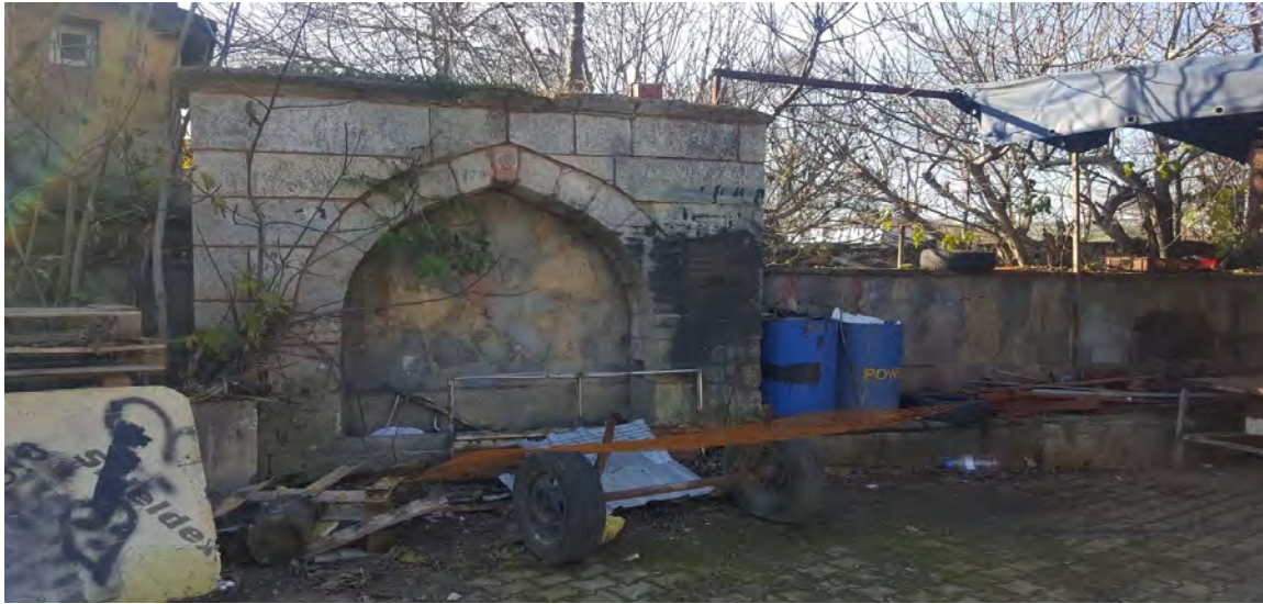
Figure 6: The dismal condition of the old Ottoman Fountain in Dursunköy.
